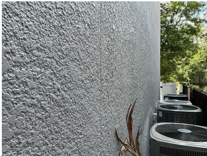
10. View of the AC units along the side of the building.
