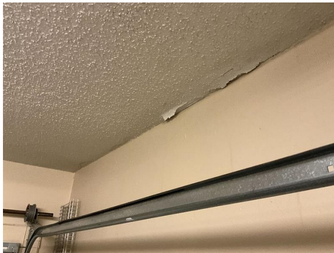
12. View of spalling in a garage popcorn ceiling.
