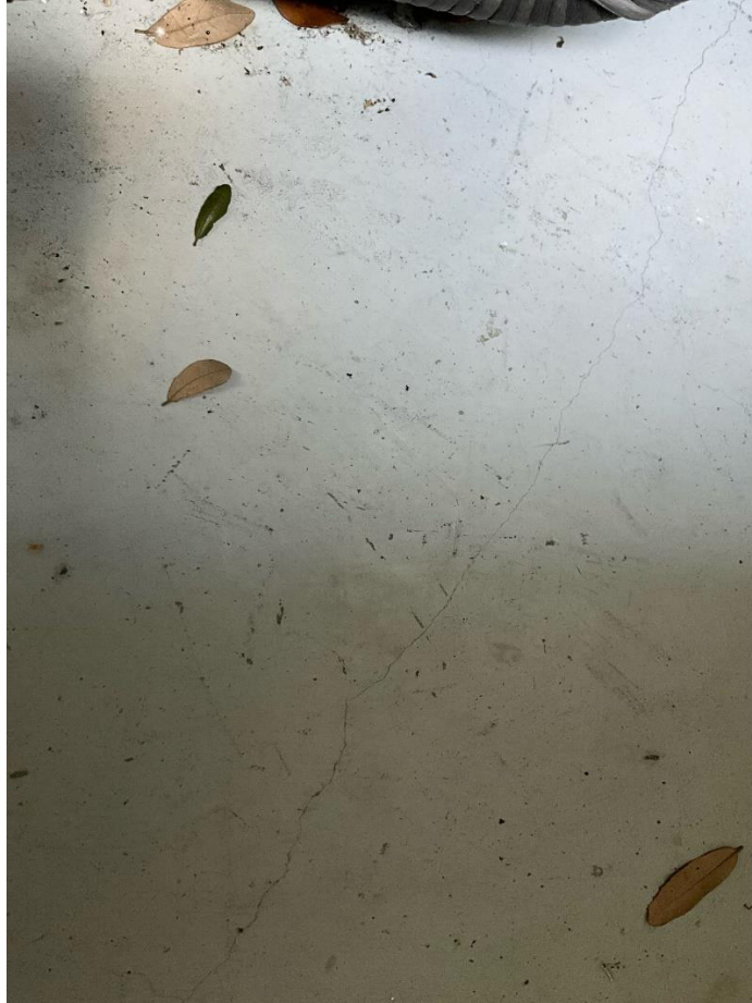
11. View of minor-hairline cracks in the balcony slabs.
